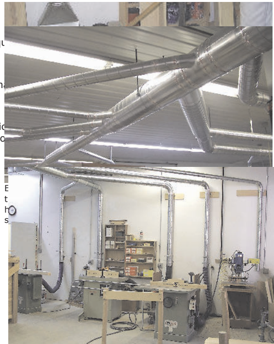
Against the wall — Yankowy installed all the piping along the wall as well along the ceiling.
