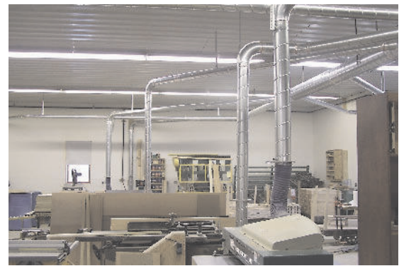
Lots of piping — For a small shop, J&J requires a fairly elaborate dust collection system to handle a single-end tenoner plus multiple planers and jointers.
